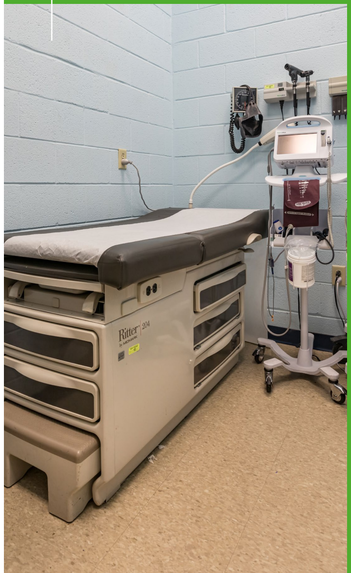
Medical Room at Alexandria Staging Facility
